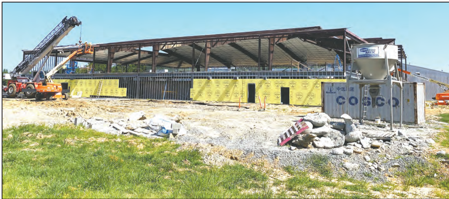
The new elementary school (top) and the new arena (bottom) are still under construction and making progress.
