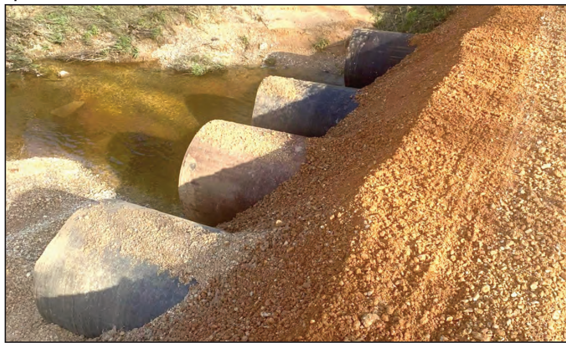
The Bradley County Road Department completed the repairs to Bradley County 45 Mt. Olive Road. The crew installed new pipes and laid new gravel on the road.
