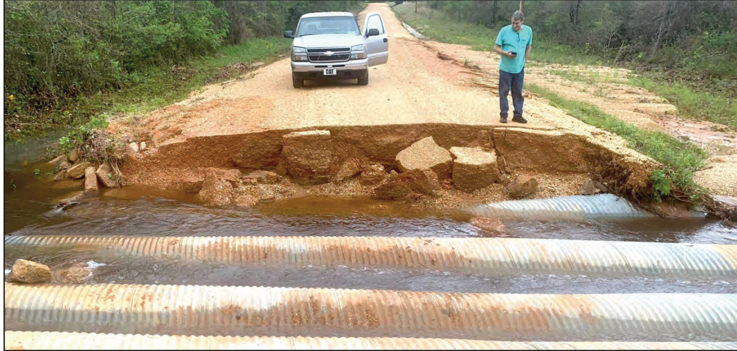
Part of Bradley County Road 45 near the Mt. Olive Community was washed out during the rainfall over the weekend. Raymond Quimby of the Bradley County Road Department surveyed the road damage.
