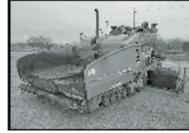
DN3642 '21 Voage Super 1700-3 conveyor
